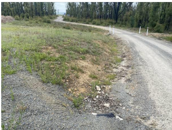
Plate 15: 50 m / 500 m range access - typical example of well-maintained access tracks - example of weed outbreak (4788).
