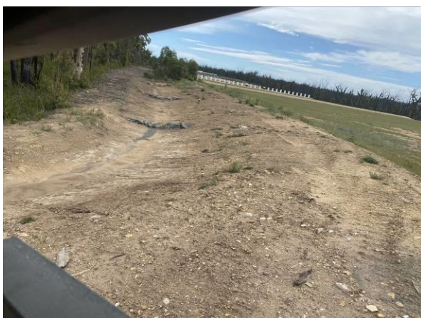
Plate 9: 500 m range - swale and sediment traps in good order with minor sediment accumulation (4724).
