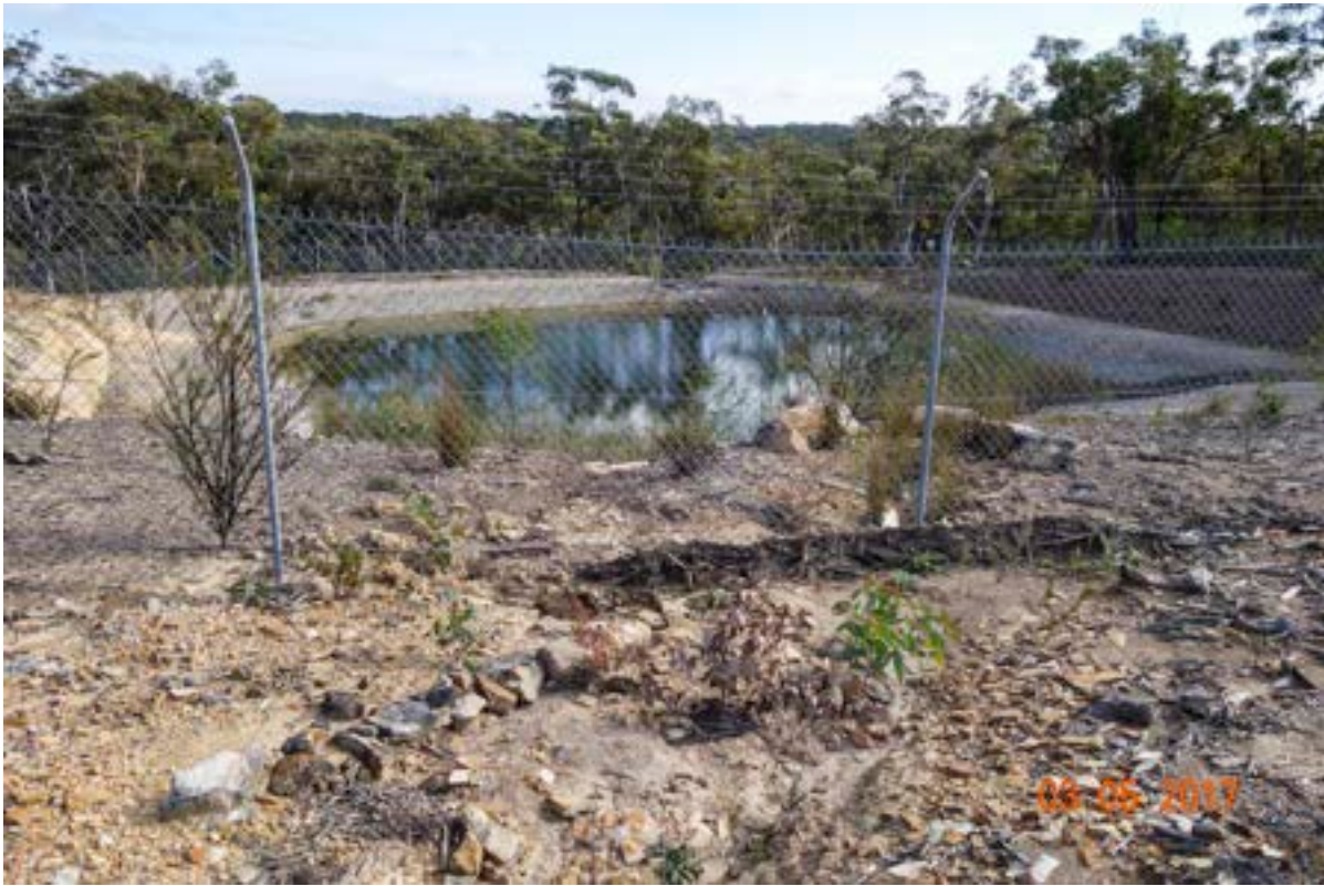
50m range: Retention pond viewed from SE side, showing erosion and debris piled against fence.
