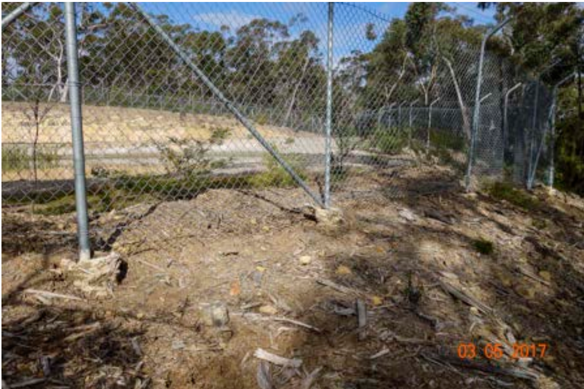
50m range: Retention pond security fence on NW side, showing erosion of fence footings.
