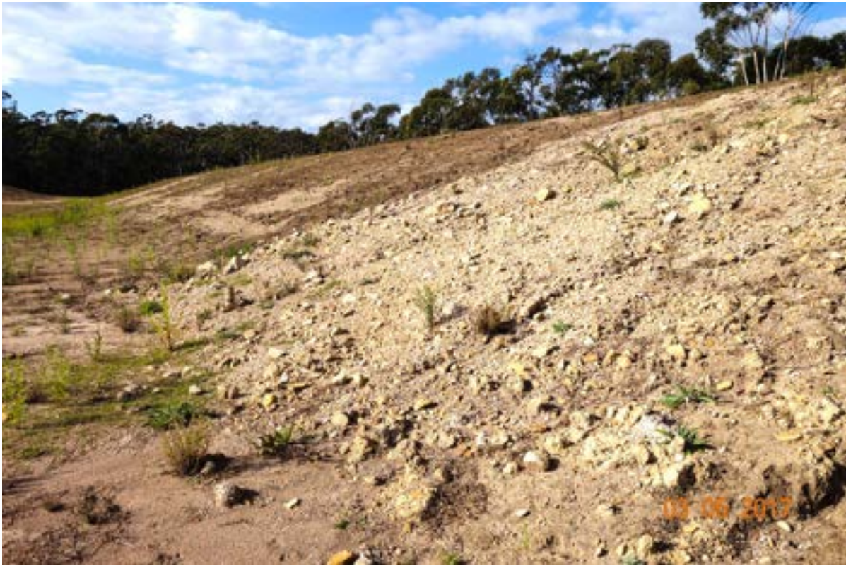
50m range: Inner slope of SW batter with slope failure and weeds.
